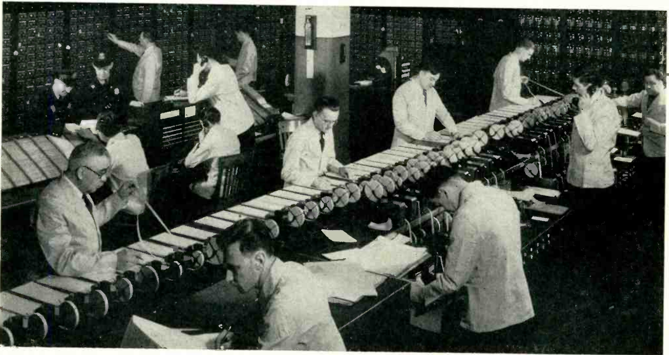
Central station in which alarm and supervisory signals from subscriber's premises are received and recorded
