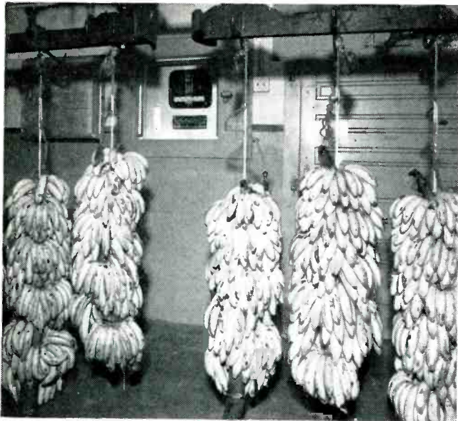
FOOD INDUSTRY Banana-ripening temperature is regulated by electronic controller on back wall, using vacuum-tube action to position steam valves accurately. This type of device indicates but does not record
