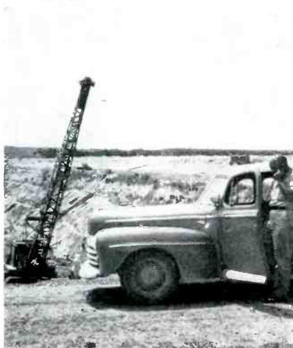
Superintendent in charge of construction of Medicine Creek Dam, George Stiers uses two-way radio in his car to call for reinforcements
