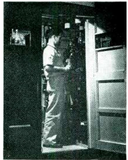
This 120-kva rectifier unit supplies plate voltage to all power amplifier tubes from the final down to the 250-watt stage
