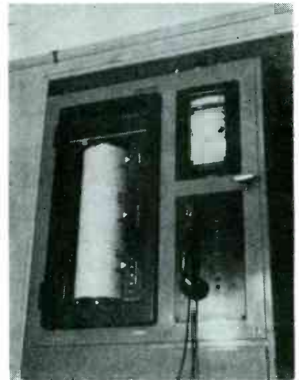
Control panel and Rittmeyer transmitter installed in the pump station
