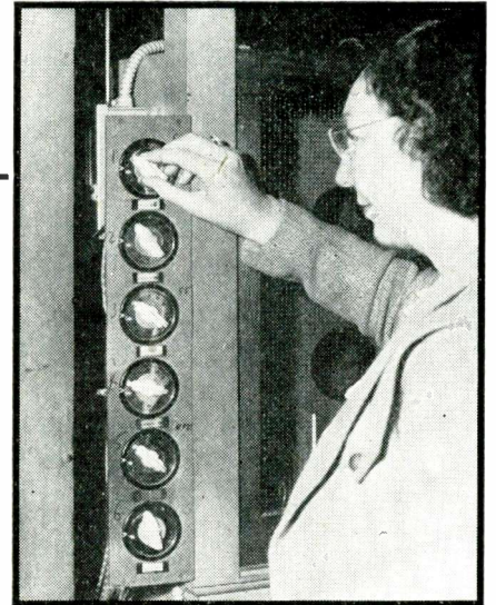
Six automatic time-switches are mounted on a vertical panel
