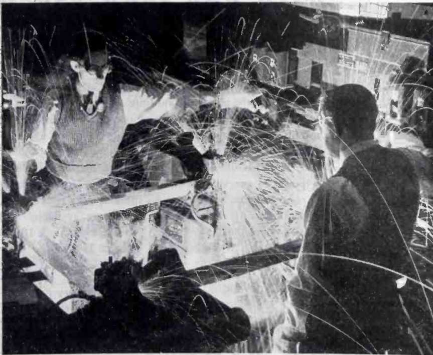
Four simultaneous flash welds are made with this four-cornered machine which fabricates 150 metal frames an hour from metal strips 0.05 inches thick. A 20 kva transformer is located at each corner and controlled by an electronic welding cycle control
