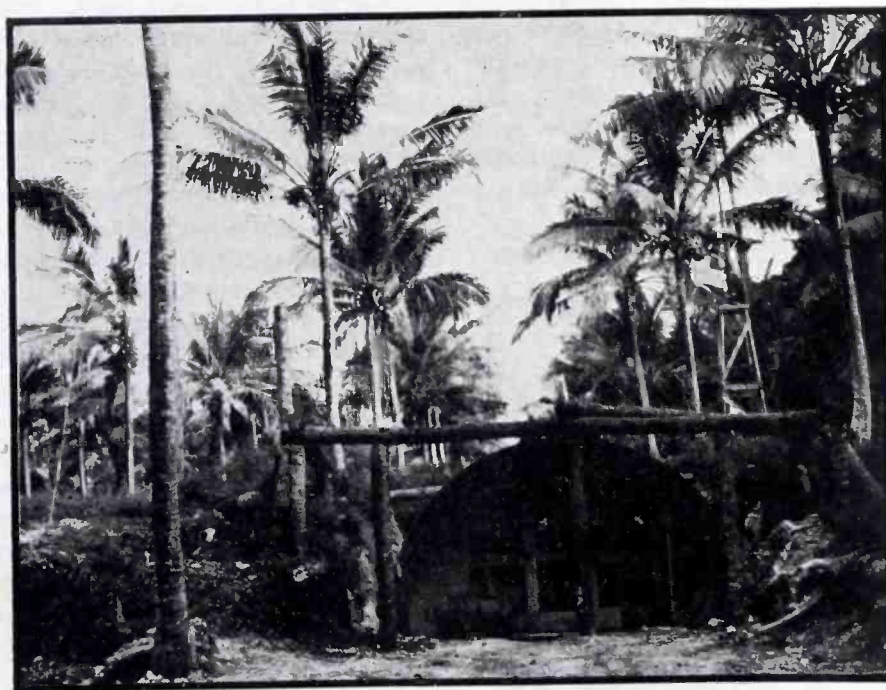
A complete airways radio station, serving aircraft shuttling over long water-hops in the South Pacific. A gasoline generator may be seen at the left of the hut and an antenna at the upper right
