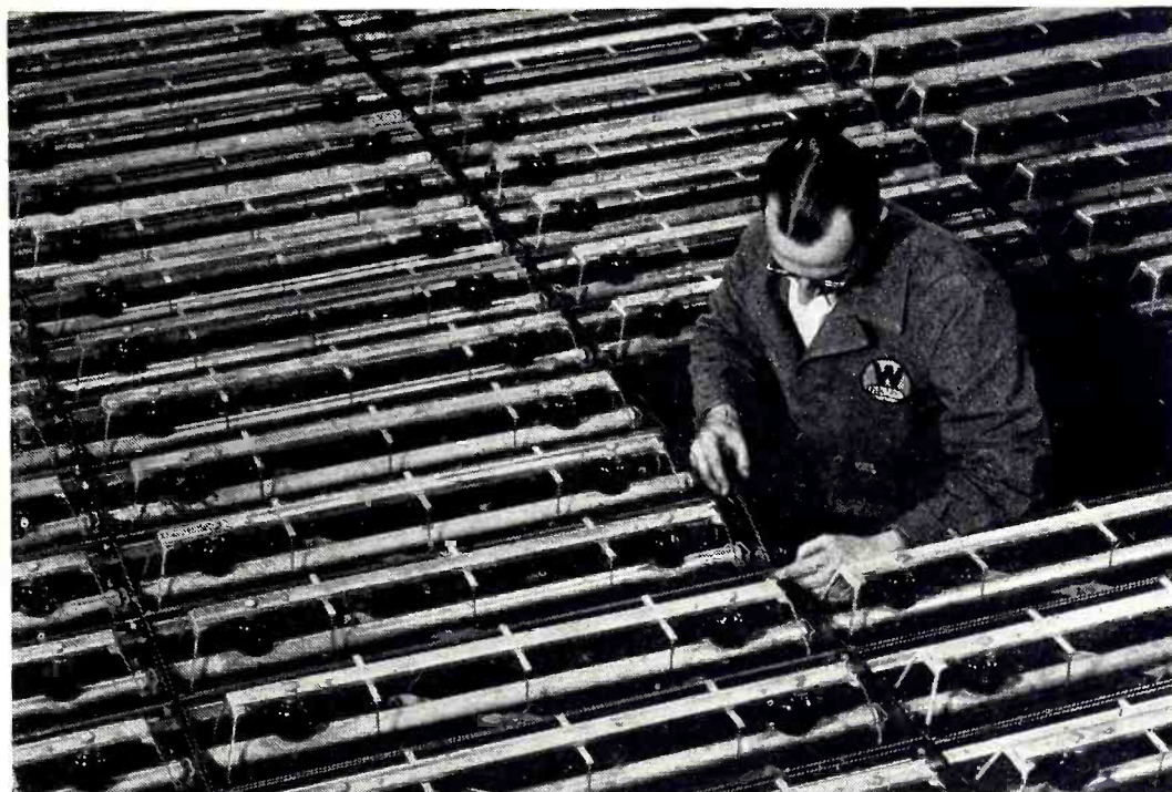
DUST —Electrostatic precipitators designed to rid air of dust and dirt use electronic principles, are more efficient than mechanical filters
