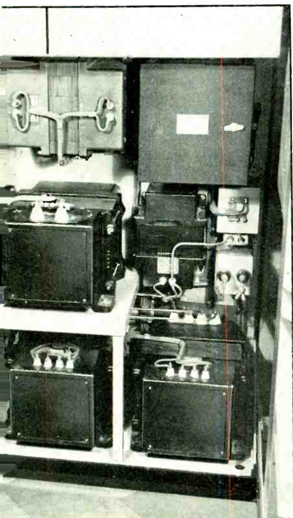
AmerTran Transformers used for the grid bias rectifier at WABC.
