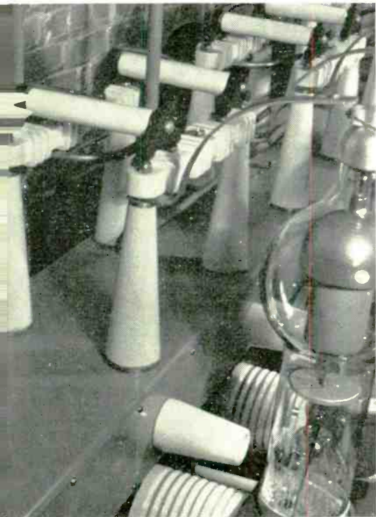
Stand-off insulators of Lapp electrical porcelain installed in the hand-switching system for the spare rectifier tubes at WABC 50 Kw transmitter.
