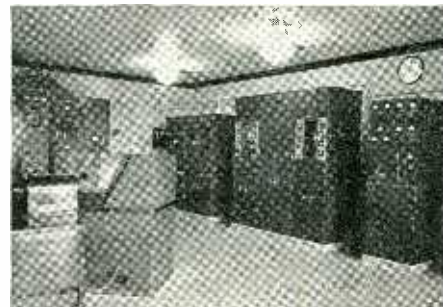
Transmitting equipment of the Kansas City Police Dept.
