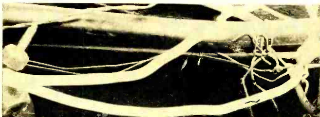
Another example of faulty power-line installation where telephone or audio lines are not shielded from the power lines.
