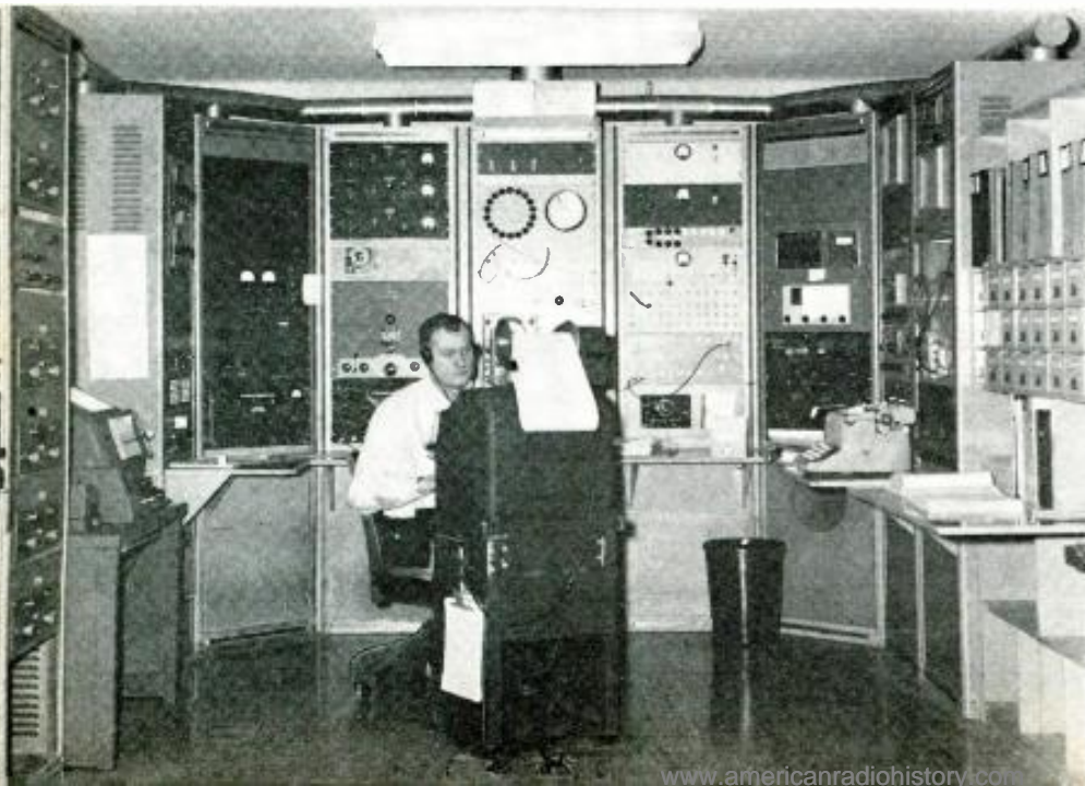
Fig. 1. Monitoring console of the Chillicothe, Ohio FCC monitoring station. Technician is contacting other stations by teletypewriter.
