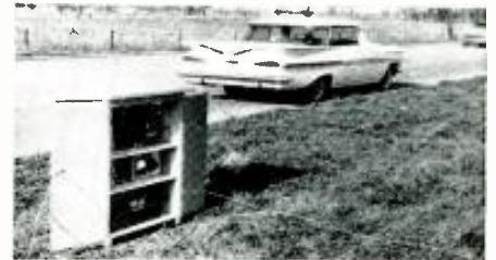
Roadside equipment in waterproof housing.
