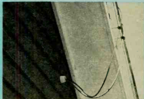
Seen from outside (below) coax and cable form drip loops outside attic; plastic tube goes through wall.
