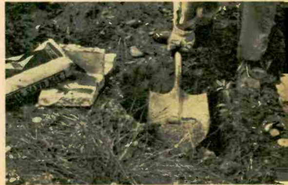
Fig. 5—Mast must rest on firm base. Here, hole is dug for ready-mix concrete (bag, left). Broken block or bricks reduce amount of concrete needed.
