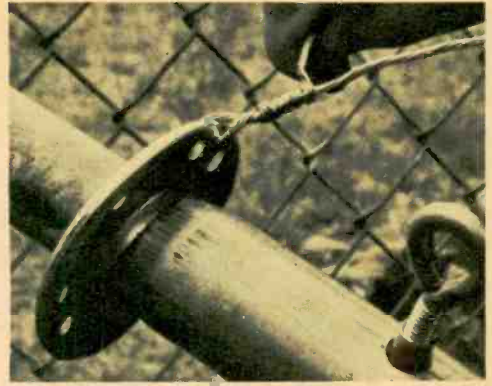
Fig. 4—Attach guy wires to rings on mast. Eye-bolt (right) holds sections during erection. Cotter pin (not visible) through mast locks sections.
