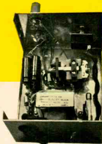
Turning telephone dial shorts J1, J2. This causes RY1 to close and apply 125 VAC to J2, J3, which rings all other phones that are connected on the line.
