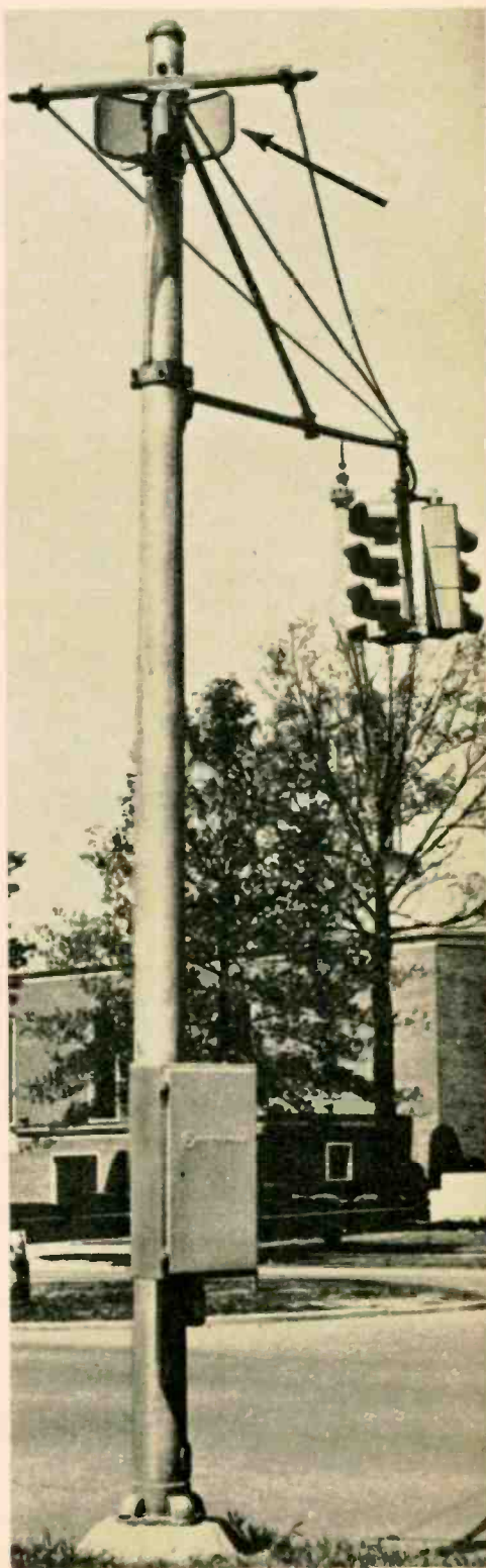
RADAR LIGHT —If it weren't for the traffic light attached to it, this pole might be a mast transplanted from a ship, complete with a radar screen. But it's really a radio-controlled traffic signal at a street intersection in Detroit. The "radar" screen (arrow) is an antenna that picks up signals from a master control center to change the lights.
