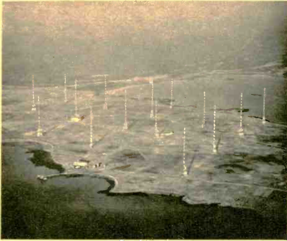
A forest of towers occupying a whole peninsula marks Navy's new two-mega-watt station, NAA, at Cutler, Me. Station's huge VLF antenna is supported on 21 towers up to 900 feet tall. Seventeen appear in this picture. Ships as far away as the Mediterranean receive NAA.
