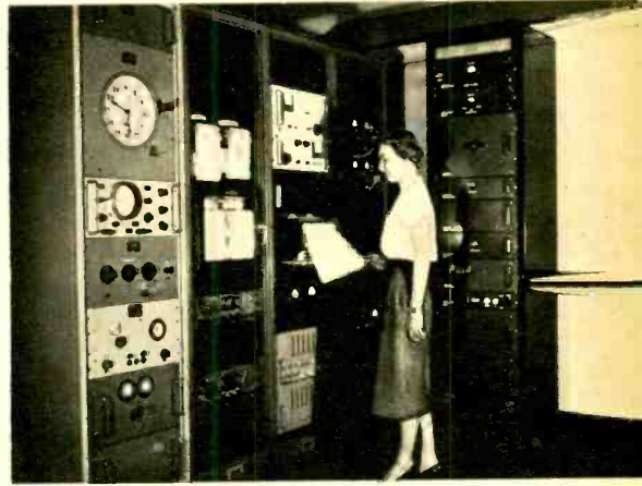
Control room with quartz-crystal clock (left) at NBA, Navy time station in the Canal Zone.
