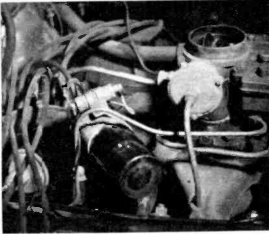
Capacitor mounted on coil bypasses primary circuit. Lead comes from ignition switch.
