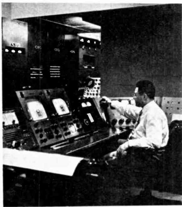
This CBS-TV transmitter operator not only controls his station's signals at the transmitter site, but must be prepared to make any necessary equipment repairs. Note scope.
