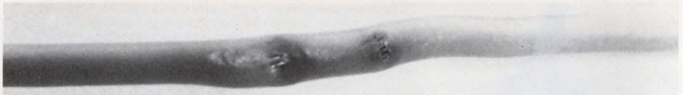
4. Exposed insulated wire can short to the equipment frame due to "cold flowing" of the insulation. Pressing,
