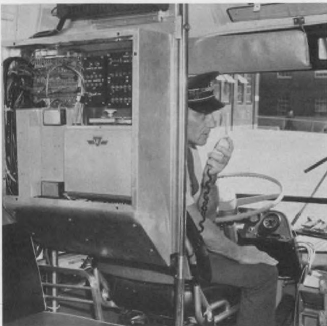
Control center in Toronto's projected communications and information system will query each of the city's transit system vehicles 10 times a second for its location
