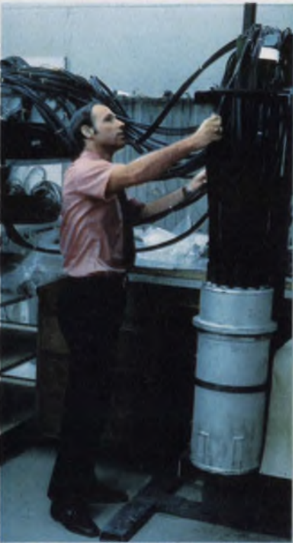
Electrical penetration conductors at Gulf take data from sensors inside a reactor's core through the containment wall to a display.
