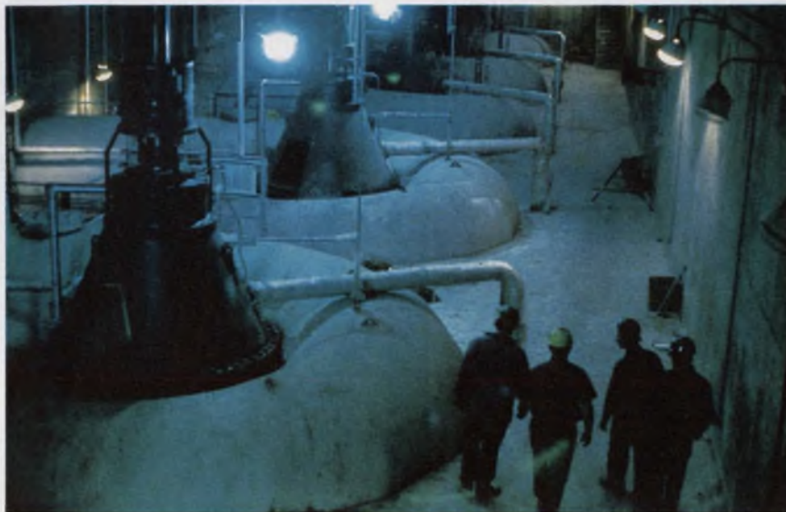
A computer displays diagnostic data from thermocouples on these giant pumps at the Commonwealth Edison plant in Zion. The pumps pull in 1.5-million gallons of water a minute from Lake Michigan to condense steam.
