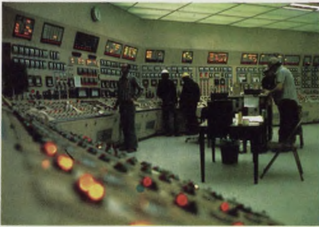
Control room at Commonwealth Edison's Dresden reactor in Morris, Ill., was built by General Electric. It displays data from sensors throughout the plant.
