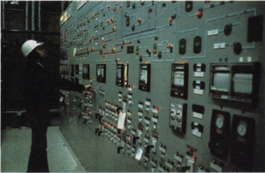
Waste disposal panel at the Commonwealth Edison plant in Zion collects data via Geiger-Mueller sensors from radioactive liquids throughout the plant. If preset limits are exceeded, the panel halts the operation.
