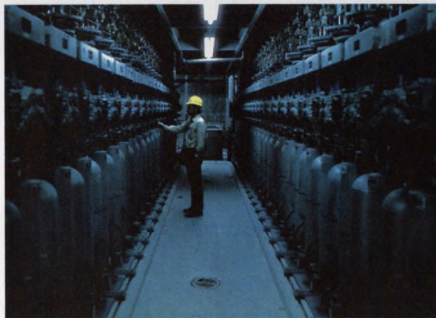
Hundreds of electronic sensors feed signals to these accumulator tanks of nitrogen. If conditions call for it, one or all of the tanks will release gas to insert the fuel rods into the core and shut down the reactor.
