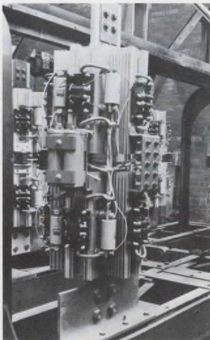
International Rectifier's diodes have replaced ignitrons in this caustic chlorine cell at Dow Chemical.
