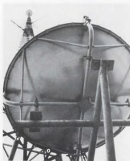
Many microwave towers like this one would be needed to provide nationwide broadband communications.
