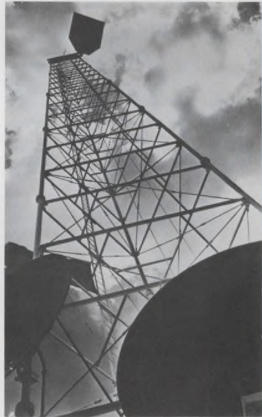
A private-line microwave net formed by hundreds of towers like this is being planned by Microwave Communications of America, Inc., and its MCI affiliates. The reflector atop the tower directs energy from the dish at lower right to the next station down the line.
