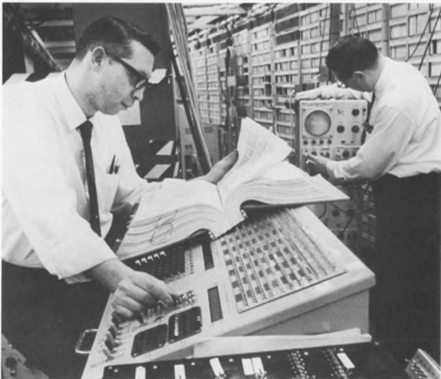
Master control center for New York Telephone Co.'s electronic switching system, one of five in the city. It handles 40,000 calls an hour and serves about 10,000 telephone customers.
