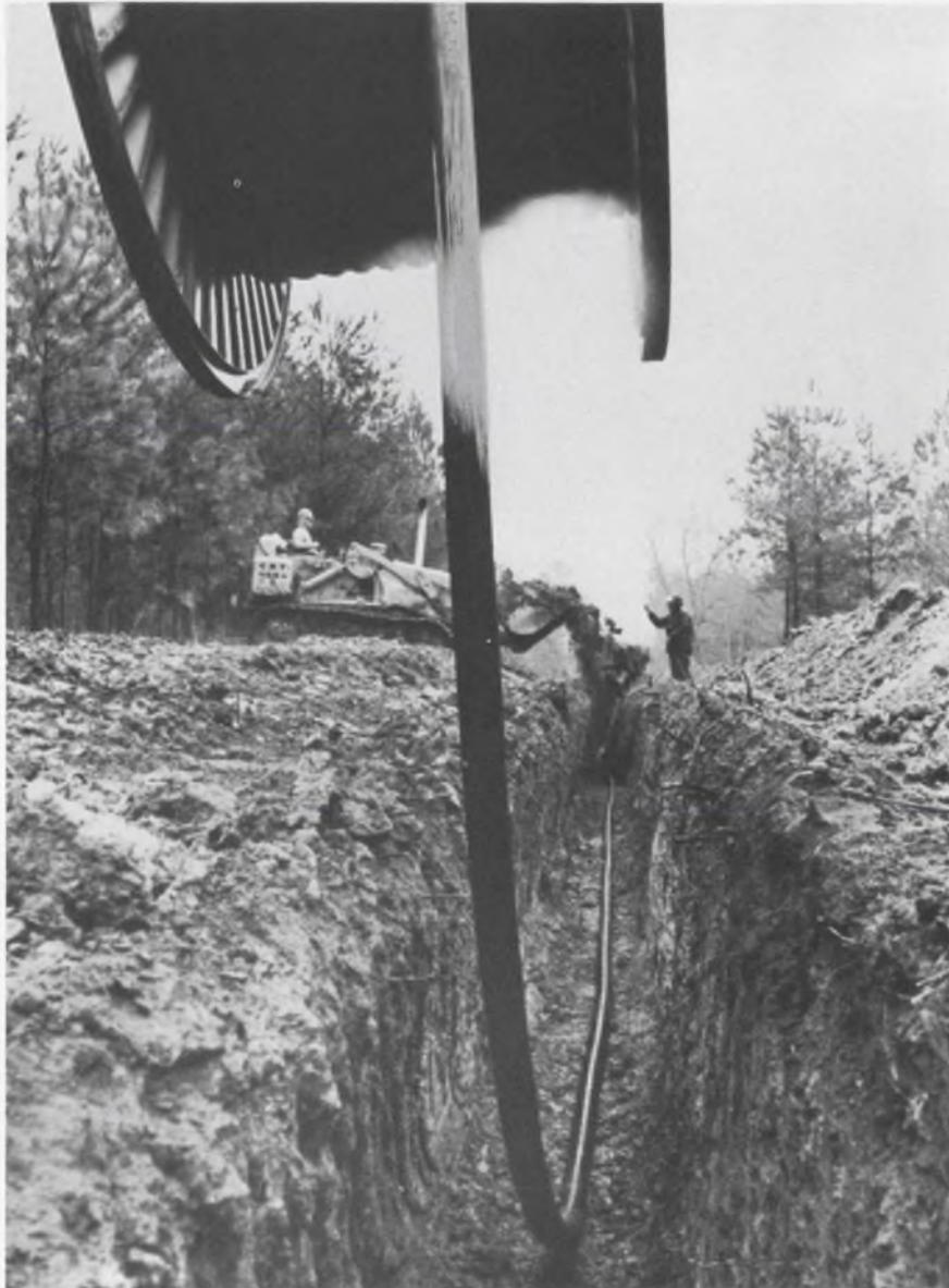
Long Lines cable —part of network of 300,000 interstate telephone circuits. The cost per circuit mile is now down to $12.00.
