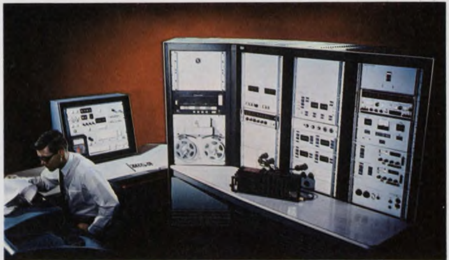
Airlines are increasingly going to computer-controlled test systems to check out their complex avionics equipment. Bendix Corp.'s test system shown above is the subject of Wescon paper 21/3.
