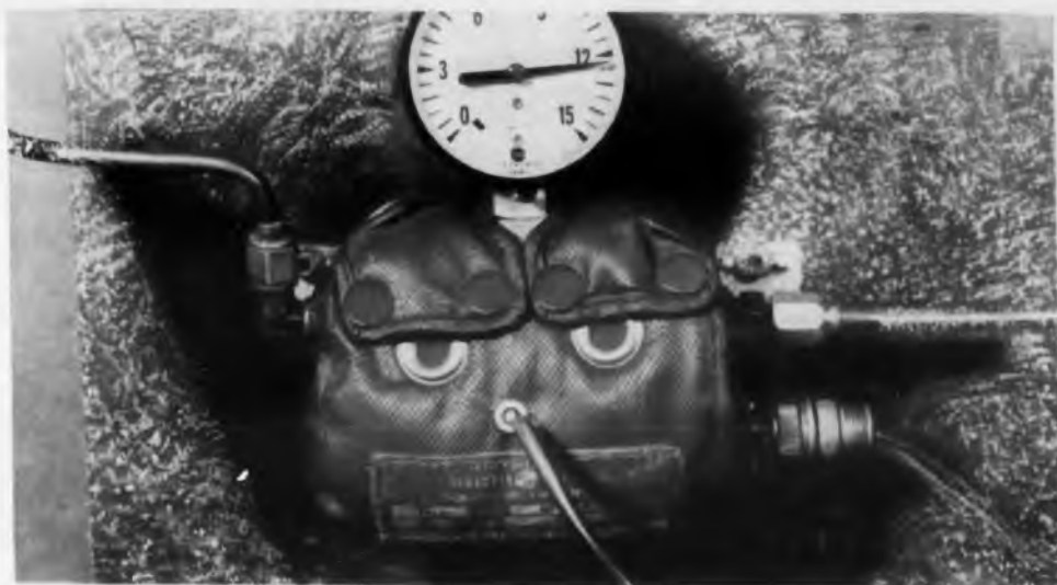
SPECIAL HEATING unit custom-designed and delivered by G.E. in 5 days enables stock valve to function properly, saves customer time, money.
