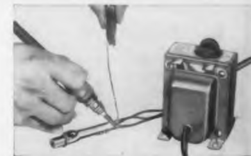
Soldering large telephone jack with Thermo-Tip Resistance Soldering Tool and low voltage Ideal power unit.
