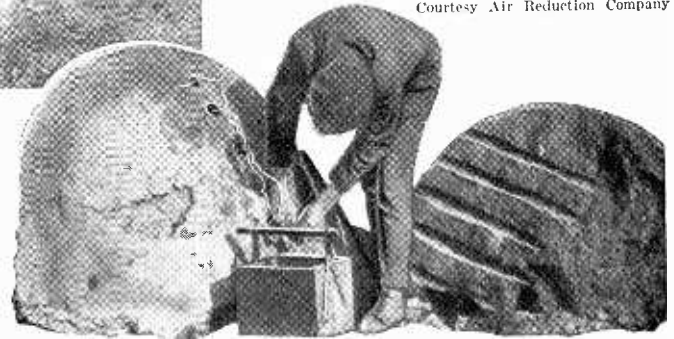
Preparatory to blasting a skull, holes are burned into it with pure oxygen delivered by a 1/4 inch gas pipe.
