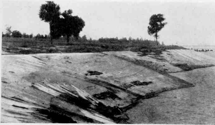
Revetments are also made by paving the surfaces of prepared slopes with concrete.
