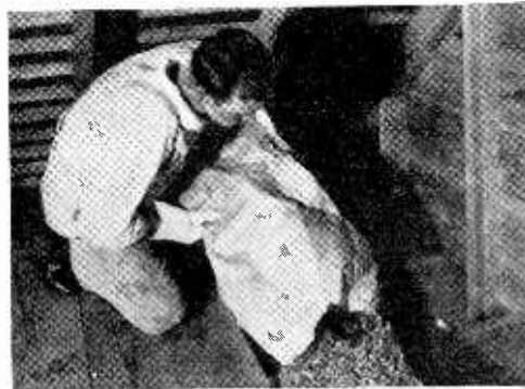
Top floor ceilings are readily insulated with fillings of rock wool. (Johns-Manville.)
