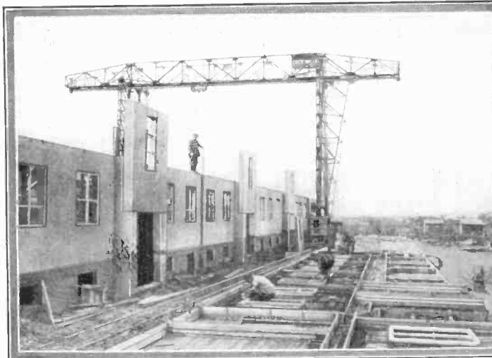
German ingenuity has contributed much to the solution of the problem of housing in congested districts by developing the unit system of home construction. Complete homes may be finished in one day, as shown above, where pre-formed concrete sections are placed on concrete foundations.
