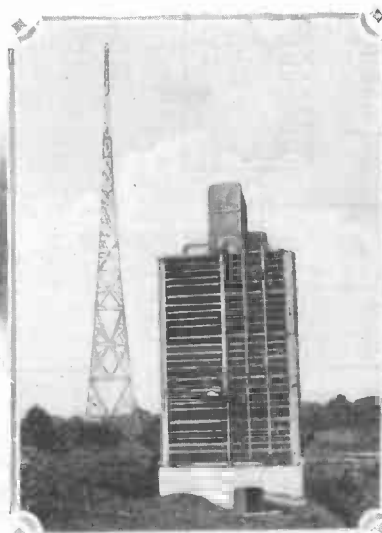
Above: The water cooler into which the water circulating around the high powered vacuum tubes at WJZ is fed in order to remove the heat that it has absorbed from these gigantic oscillation generators.
