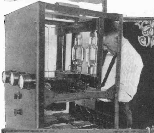
The popularity of radio broadcasting brings forth new stations every month. One of the latest is that of the Third Avenue Railway Co., New York City. The above photo shows a view of one of the twin transmitters. This station is noted for its neat layout and overall efficiency. The engineer is inspecting the 250-watt tubes which are responsible for present day broadcasting.
