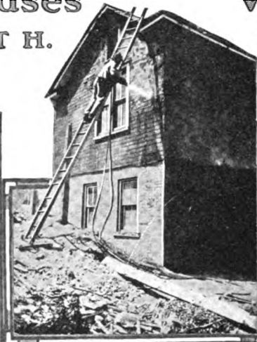
The Illustration Above Shows an Old Building Being Renovated With the "Cement Gun." After Covering the Walls With Wire Mesh to Support the Stucco.
