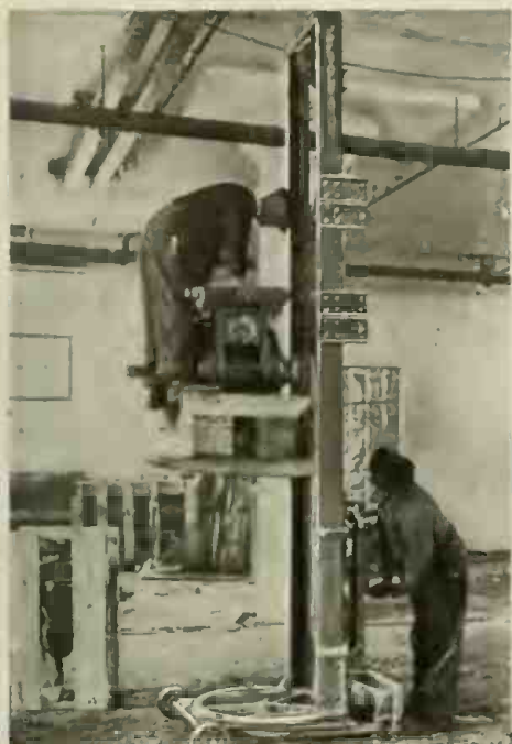
A Time and Labor Saver Which Every Electrician Will Appreciate, is This Latest Portable Elevator for Erecting Ceiling Motors.
