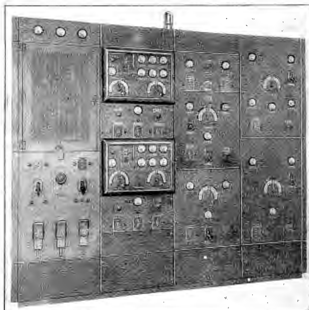
Fig. 3. This panel is one kw exciter unit, crystal controlled, for short wave transmitters and is the first unit of the short wave installation, the power amplifier unit having been illustrated in the photograph in Fig. 1
