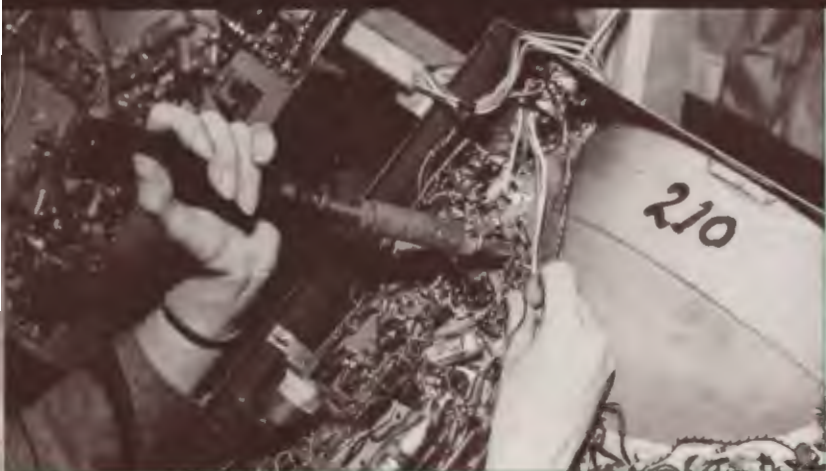
INDIVIDUAL WIRING connections are made with special care to assure lasting efficiency and guaranteed performance. Workers are highly skilled...specially trained.
