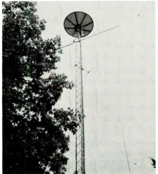
Figure 5. Dish is Parked Straight Up
