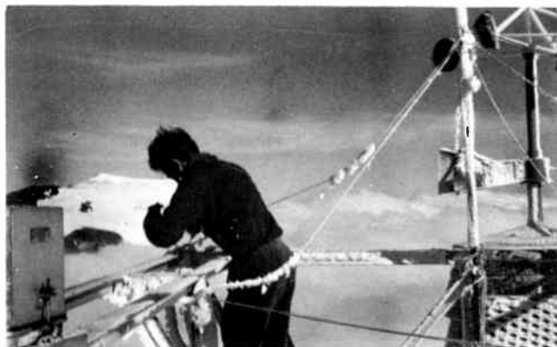
Over a mile high and still having antenna troubles! Here's the author making some last-minute repairs on frozen guy wires.
