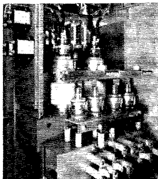
Center cubical of GATES HF-10 Transmitter illustrates husky tank circuit design for high efficiency coverage over entire frequency range.
