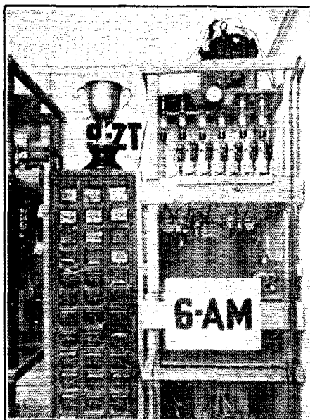
THE FILTER BANK AND POWER PANEL. The rather impressive condenser bank is not often used. It is made of many low-voltage old-style condensers and has a total capacity (with present connections) of 1/3 μf, which is ample to turn the note of this station into "pure d.c.", showing the great ease of filtration. In the power panel we have from top to bottom, 3-k.w. transformer used for Kenotron filament supply, bank of rectifier tubes, one group of high voltage transformers, some chokes, second group of high-voltage transformers. The cup and the 9ZT card are Minneapolis souvenirs.
