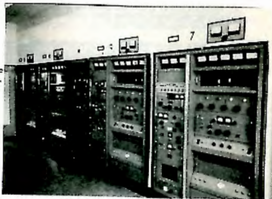
The relay transmitters for the SW link to Portugal and Spain.
