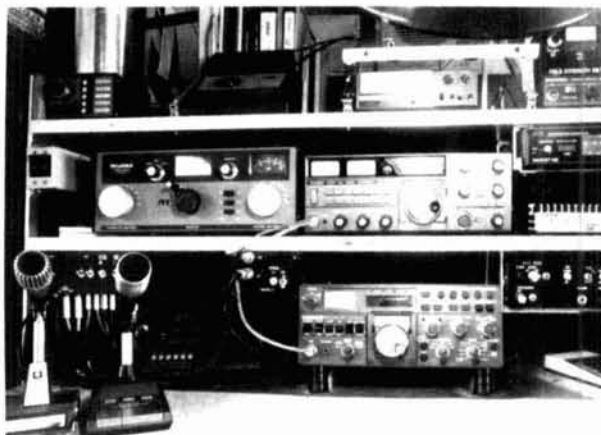
Interface box and rigs.
