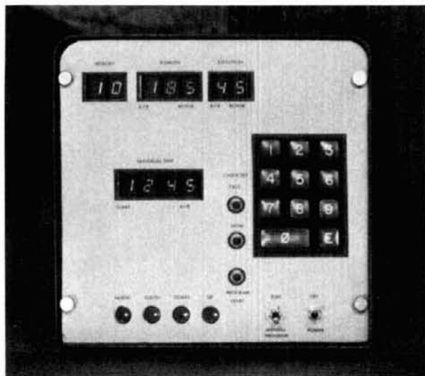
Photo A. Controller mounted in a BUD cabinet. The RUN-PROGRAM/MANUAL toggle switch shown here has since been changed to a 3-position rotary switch.
