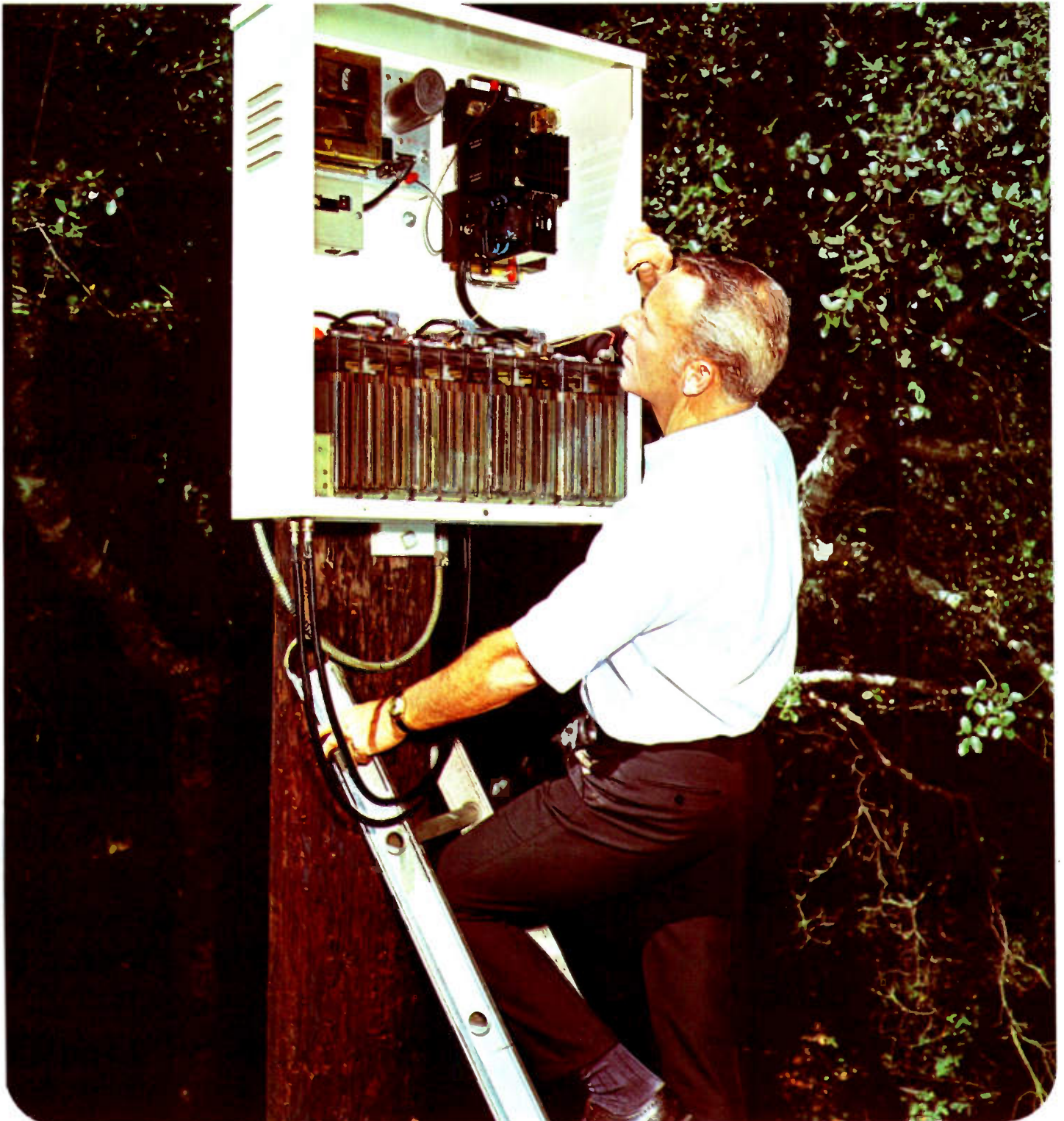
Rich Laboratories' emergency power supply receives final inspection after installation in TelePromTers' Santa Cruz, California system.
