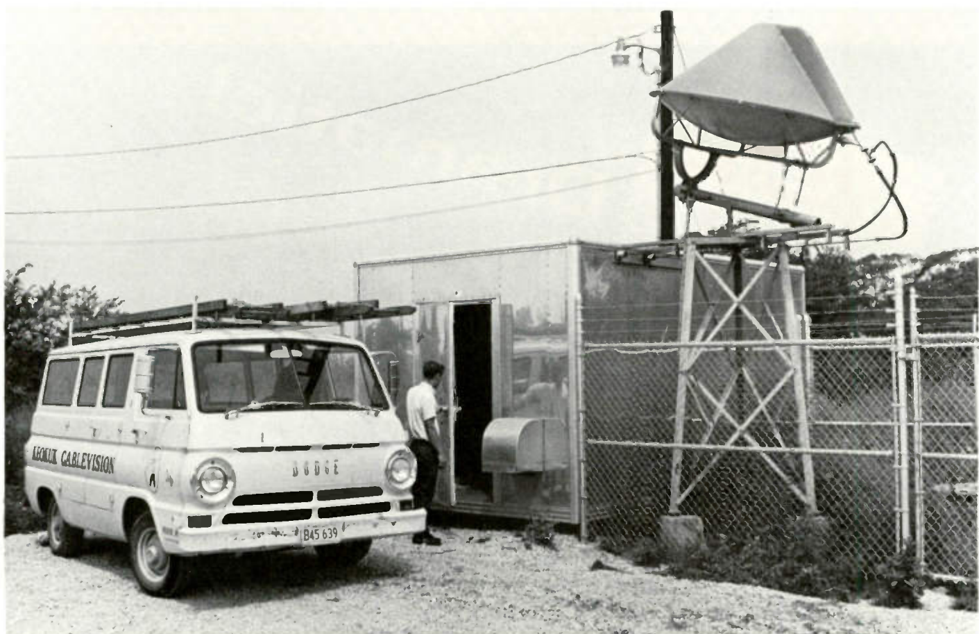
Bill Hinton, Chief Technician, Keokuk Cablevision (sister company of Quincy Cablevision) enters the microwave building at the Keokuk site. The site is the terminal point of the microwave system. Coaxial cable carries the signals on to Hamilton.
