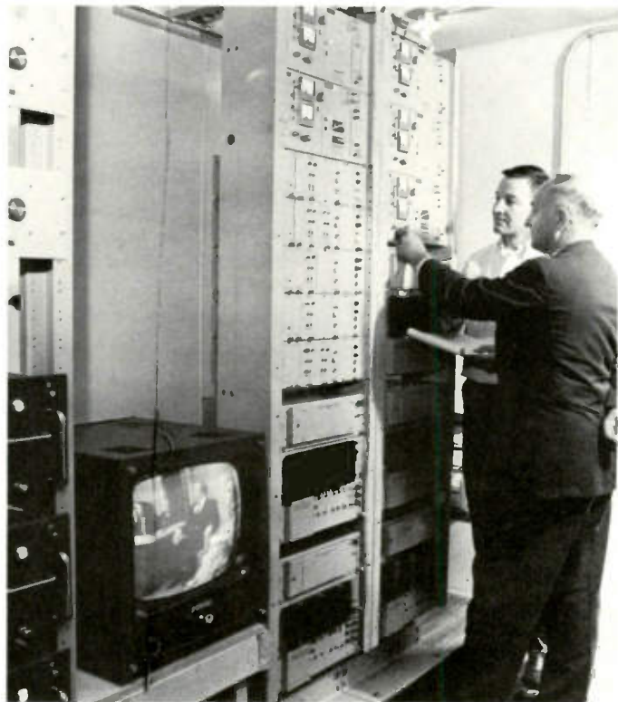
Meter readings are recorded at the Louisiana microwave radio site by Richard Ashpole, Chief Technician, Quincy Cablevision, left, and James A. Teslik, Senior Sales Engineer, Lenkurt. Signals are relayed from Louisiana to Hannibal.
