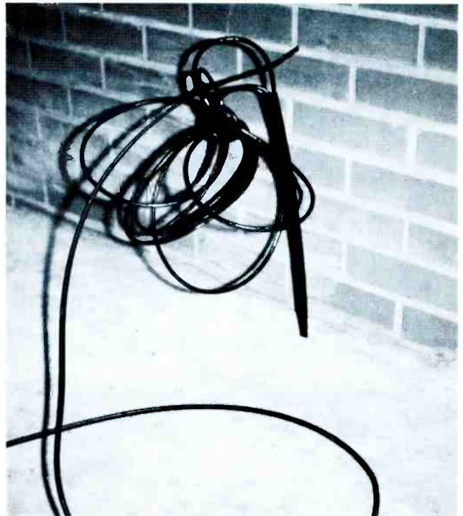
Telephone cables protrude from sidewalk and wall, creating unsightly hazard to persons using sidewalk. 75 ft. of cable is strung from this entrance across the ground to "buried cable" pedestal.
