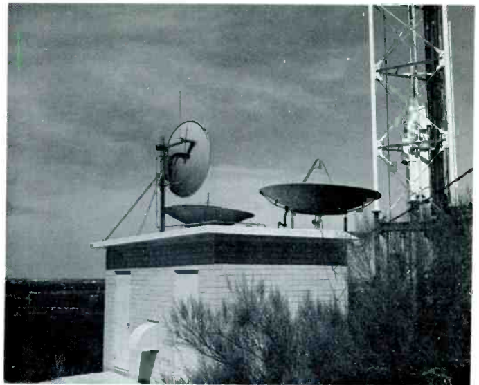
The 6 and 12 gc antenna installation at the KTBC repeater tower. The Austin television station (KTBC) permits use of its tower and site for utilization by TEMP.
