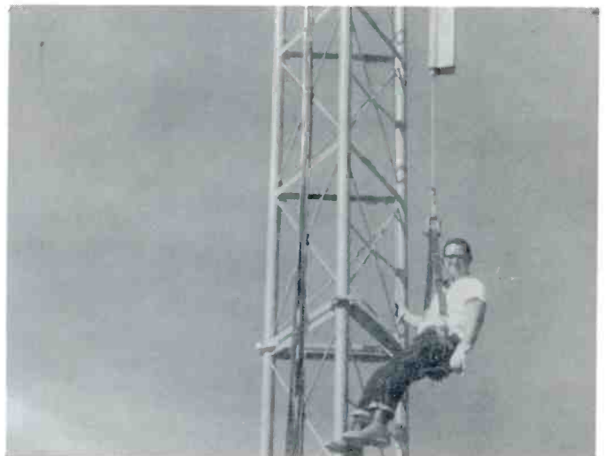
System technician taking the easy way up to finish connecting the antennas. Lift makes it up to the top in 6 minutes.
