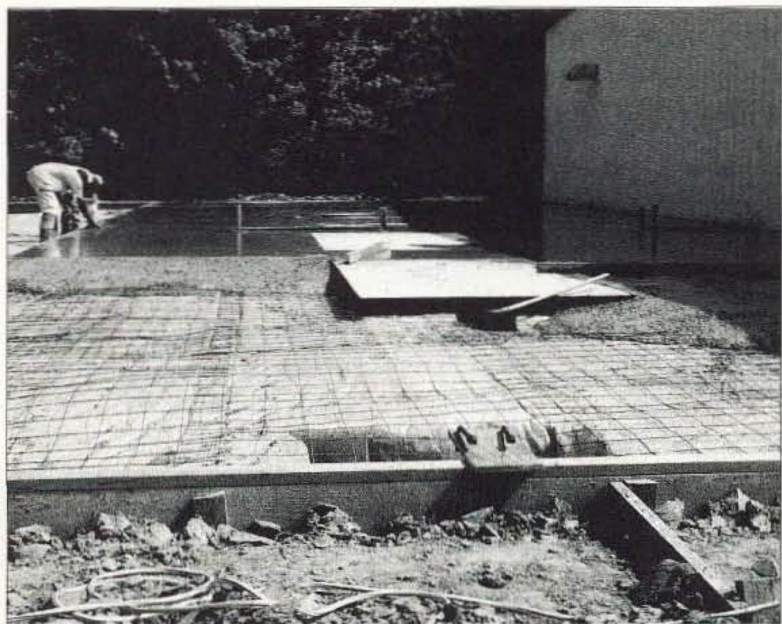
Photo A. Hy-Gain's expansion takes shape — or is this their new Rebar Ground Plane Grid?
