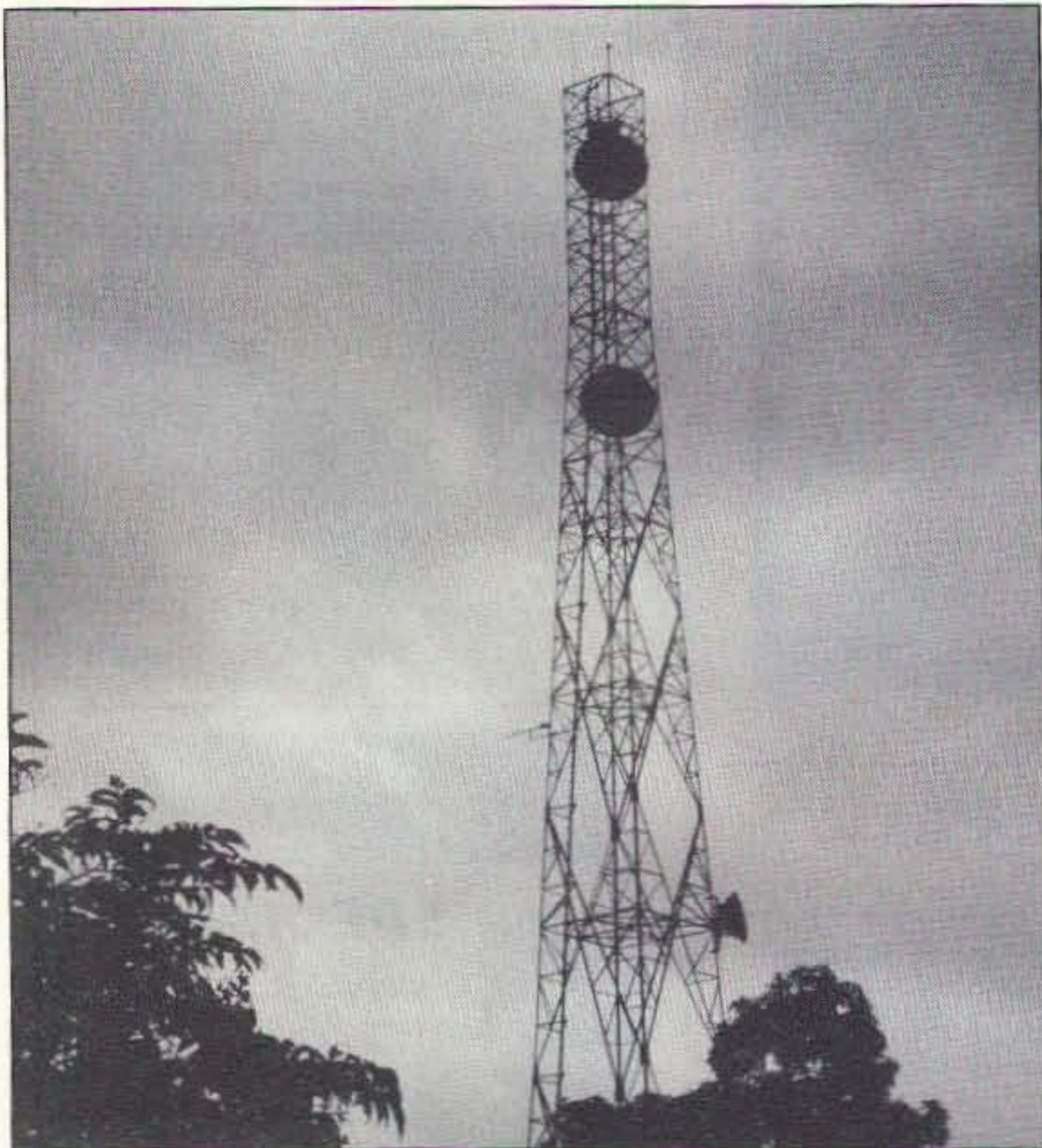
Photo C. The offending signals were being transmitted from the airport to this small yagi, halfway up the tower in downtown Freetown.
